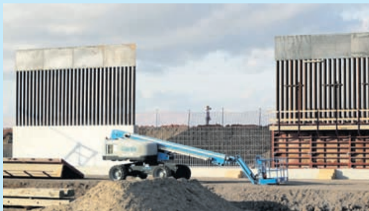
In this Nov. 7, 2019, file photo, the first panels of levee border wall are seen at a construction site along the U.S.-Mexico border, in Donna, Texas. Major construction projects moving forward along the U.S. borders with Canada and Mexico amid the coronavirus pandemic are raising fears workers could spread the sickness within nearby communities.
